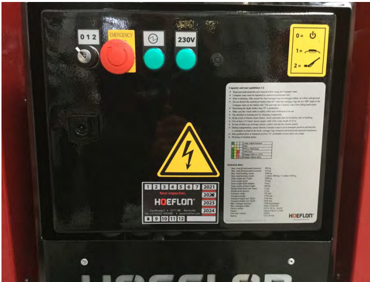
Figur 2.5 Electrical cabinet exterior
